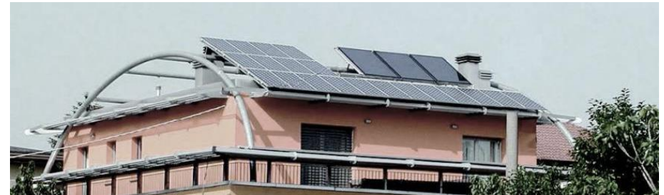
Solar and photovoltaic panels.
