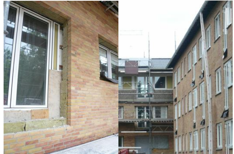
Figure: 190 mm insulation plus exterior solid standard bricks. Energy windows – aluminium – wood, 3-layer energy glass. In the panel walls: 285 mm insulation plus exterior solid standard bricks.
