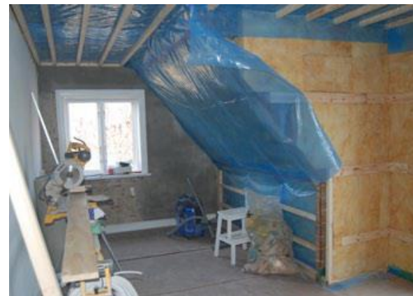
Insulation of mansard walls and lost space walls in attic incl. vapour barrier and internal insulation of the pediment
